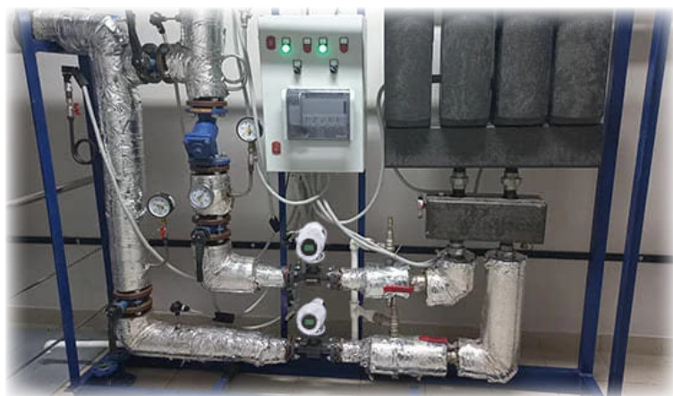
Fig. 7. Punct termic individual (PTI) automatizat
